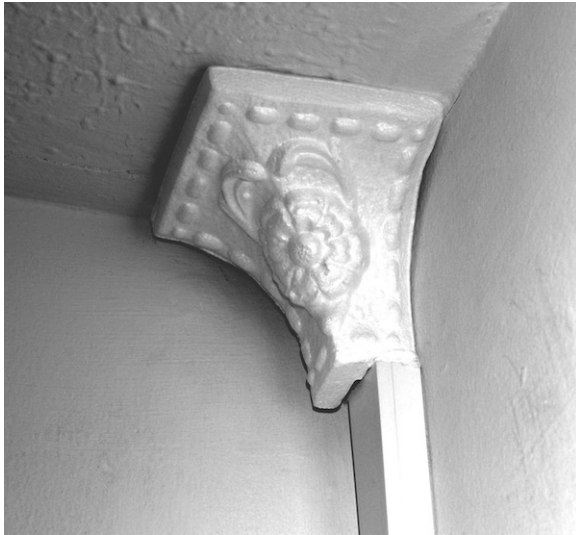
Figure 4-1. Trunking to hide the cables and a volute to (try to) hide the join.
